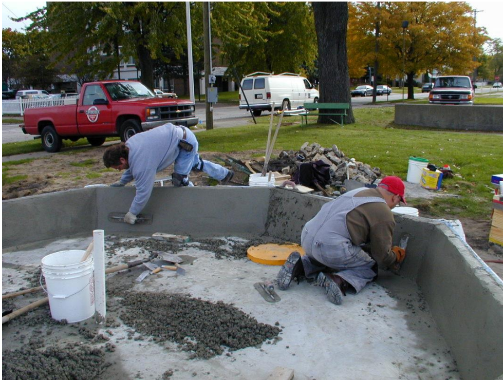
Image 09: Laying up dry-pack concrete walls within the interior of the cast iron walls for Kearny Park Fountain
