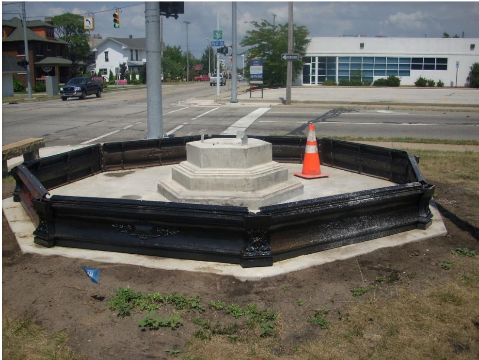
Image 07: Example of Walls in place and pedestal in place for Root Park Fountain
