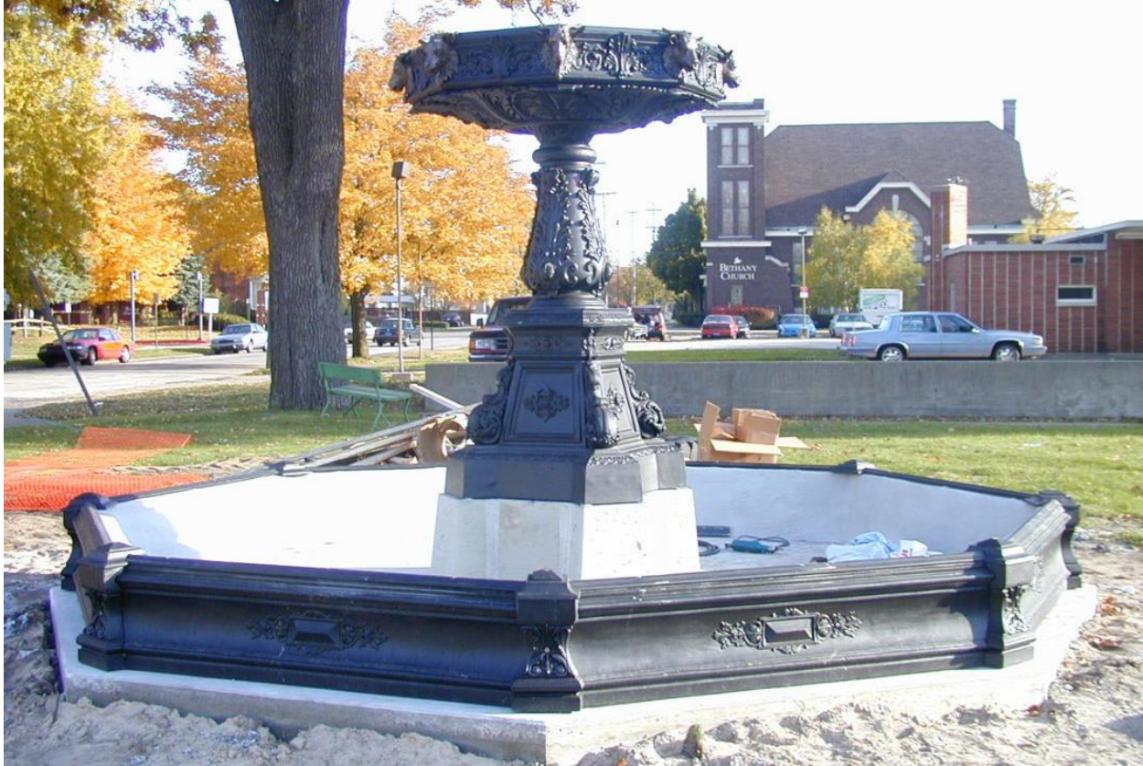
Image 10: Final install of the cast iron, waiting for application of the interior waterproof coating for Kearny Park Fountain
