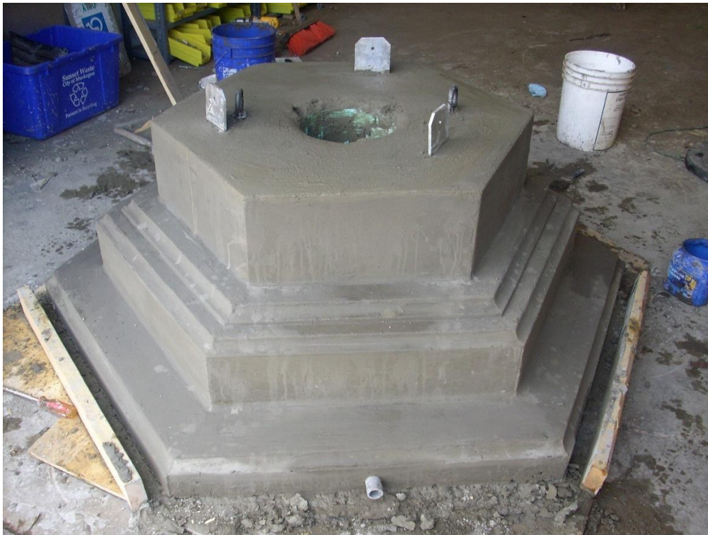
Image 05: Concrete pedestal with lifting eyes, tabs to bolt the bottom of the cast iron base to, hole through center to allow for water supply, Root Park Fountain, Muskegon, Michigan
